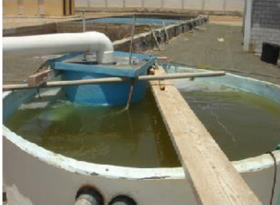
Pic-2 .The Foam fractionators
